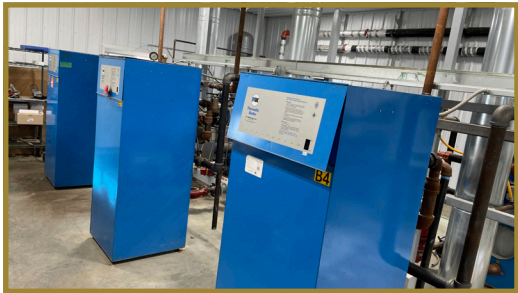
Boiler Room controls
