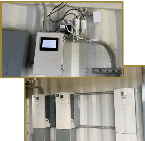
Pump Station controls
