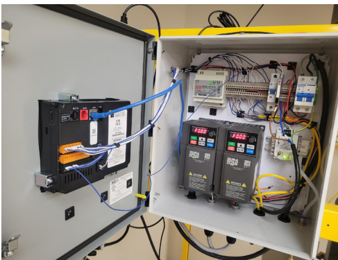
Horner X10-A in system panel
