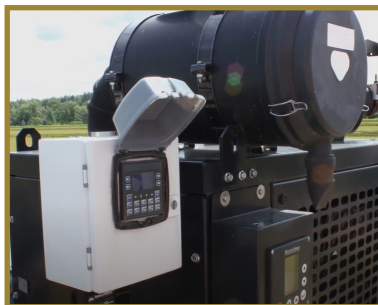
XLE shown inside panel connected to irrigation motor
