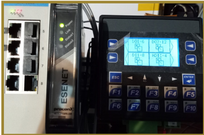
XLe in power backup system
